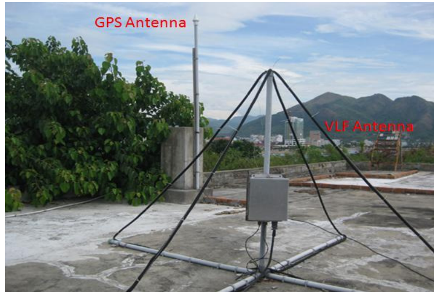
The installed GPS and VLF Antennas
