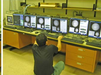
Installation of the telescope-controlling PCs and camera-controlling PCs
