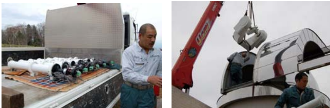
Fig. 2 Dismantlement of the original FMT at Hida Observatory for the preparation of transporting it to Peru on 10 th November 2009.
