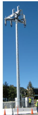
Figure 2: AT&T Cell Phone Tower at SLAC
