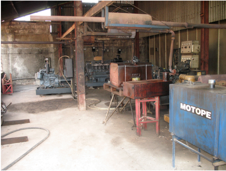
Figure 2: A building housing generators for an ISP in Guinea Bissau. The closest generator was poorly tuned and exhausted into the room, causing dangerous levels of carbon monoxide to accumulate in the work area.
