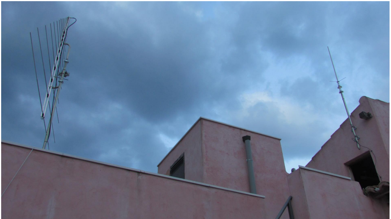
Fig. 1: New antenna installation (LPDA) in Sigüenza, Spain.
