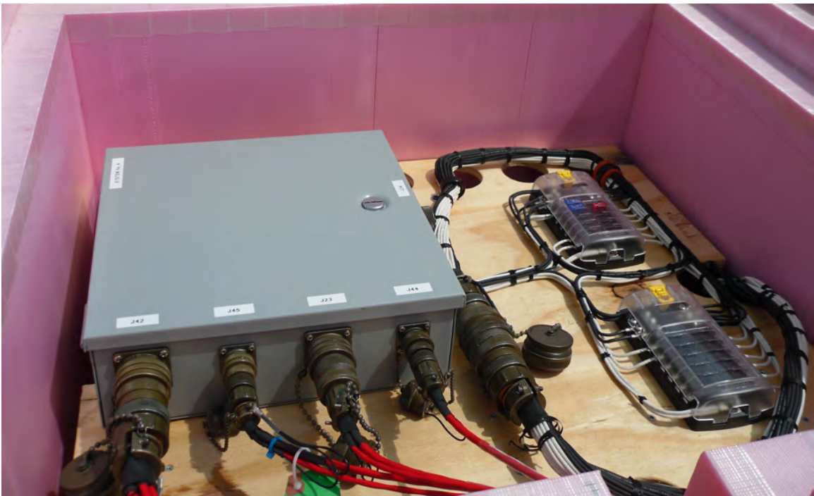
Figure 7. Power control electronics and fuses on top of the batteries.
