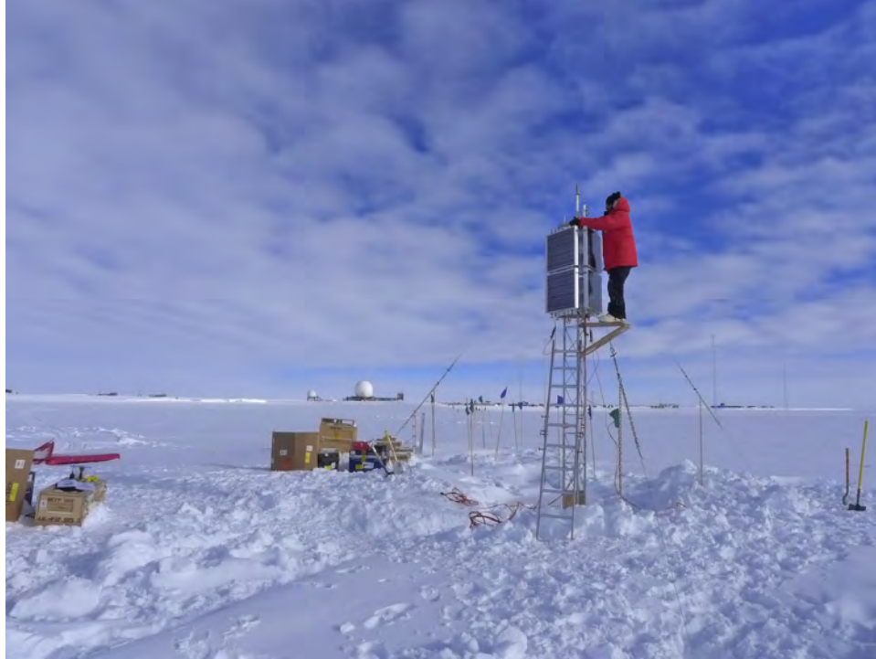
Figure 24. Majid Manteghi installing the solar panels on the tower of the AAL-PIP system at South Pole Station.
