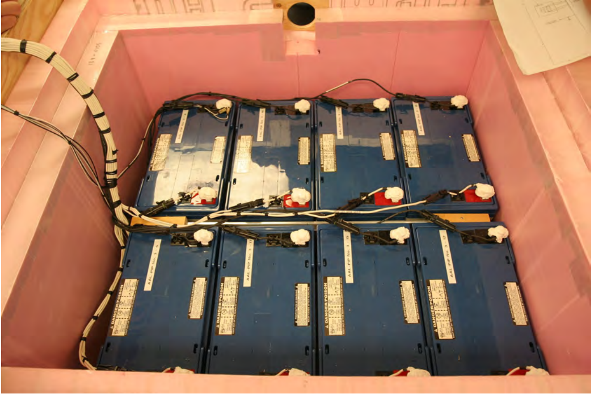
Figure 6. Lead-acid batteries in the battery box.
