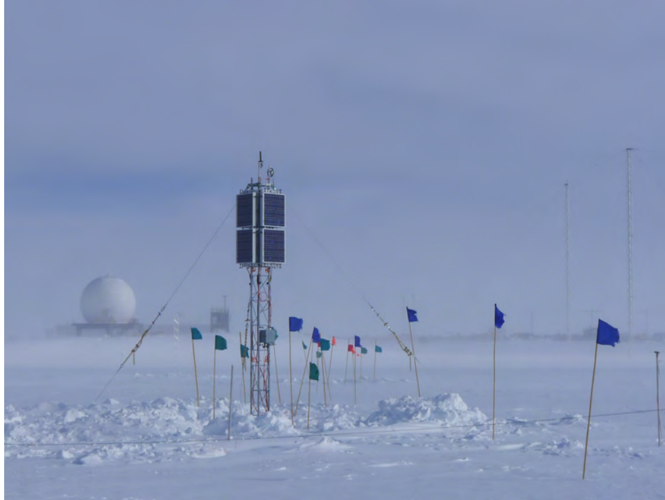
Figure 26. AAL-PIP system installed at South Pole Station.
