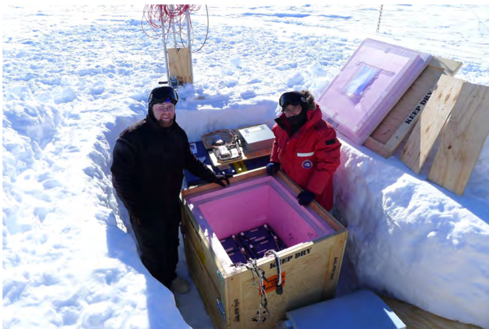
Figure 18. Joseph Macon and Hyomin Kim assembling the battery box (Sys3) at South Pole Station.
