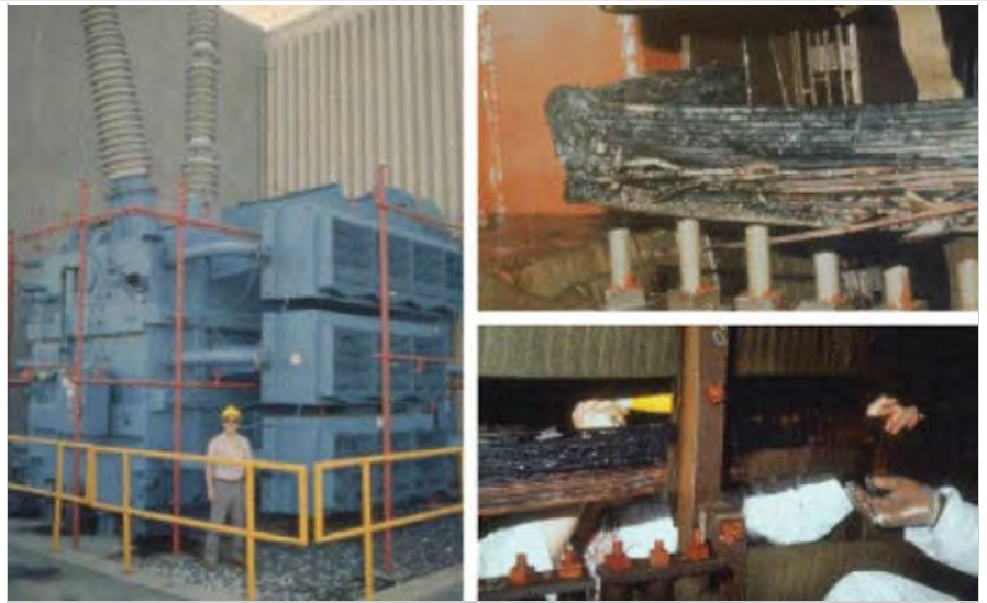
Permanent damage to the Salem New Jersey Nuclear Plant GSU Transformer caused by the severe geomagnetic storm of March 13, 1989. Photos courtesy of PSE&G. More
