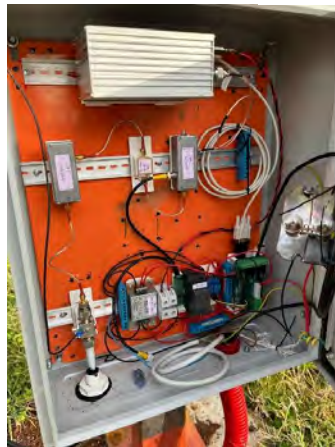
Figure 5: Complete electronics in enclosure
